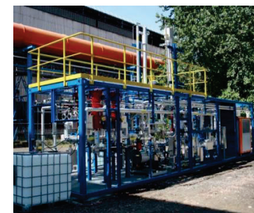
CO 2 capture unit at Arcelor Mittal Gend (Belgium) C2V Interreg project 2021
